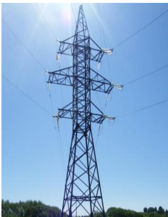
Рисунок 8.1 – Опори ЛЕП (URL: http://euroformatsteel.com/ua/service/steel-structures-for-energy-industry/steel-lattice-towers-for-overhead-electricity-lines/ )
